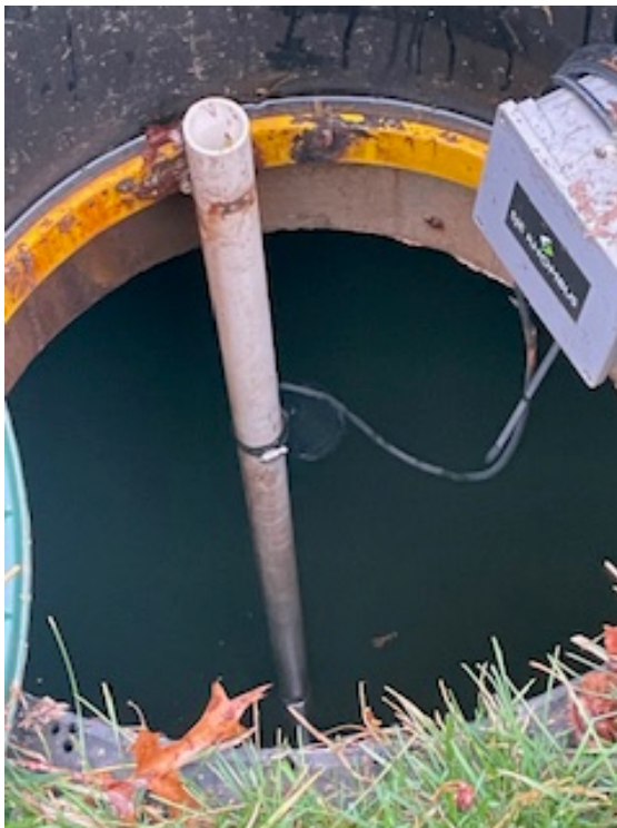
Holding tank high water alarm float
