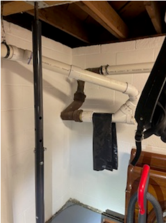
Main sewer line out basement wall
