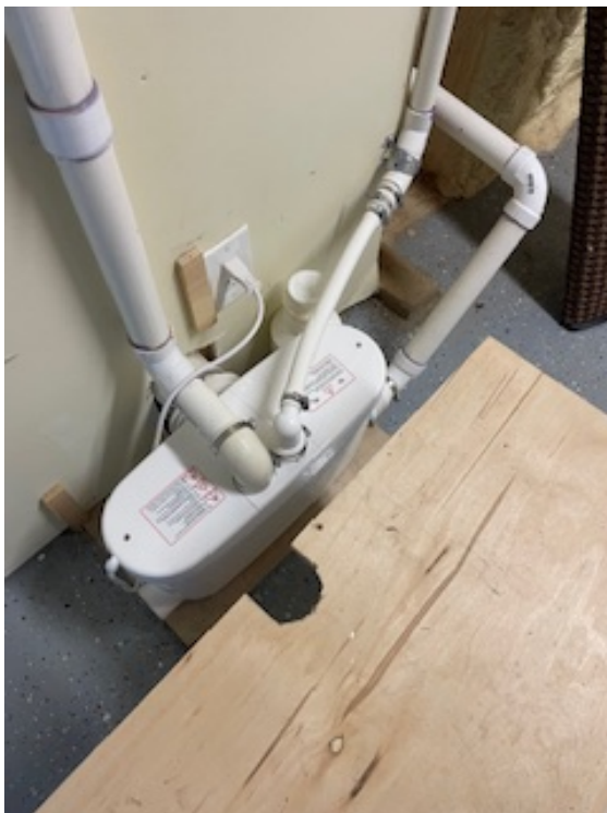
Basement bathroom pump station
