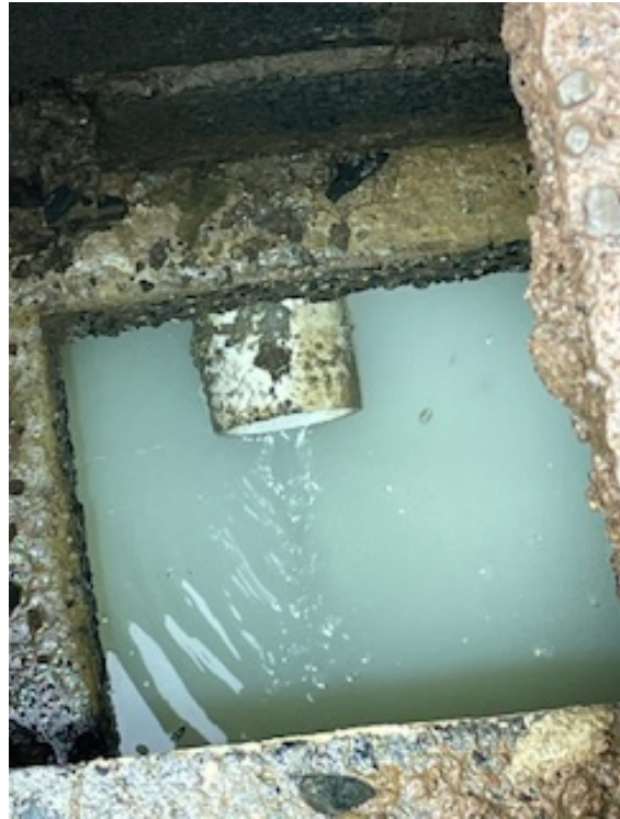
No inlet baffle in septic tank
