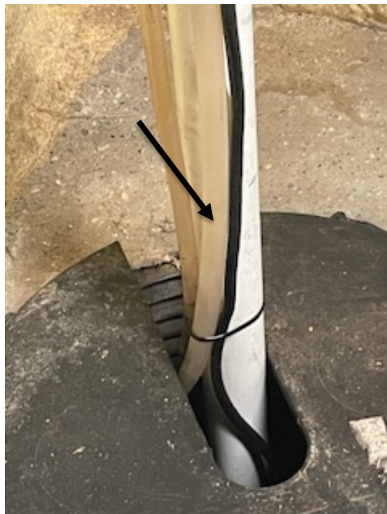
Water softener plumbed into sump pit
