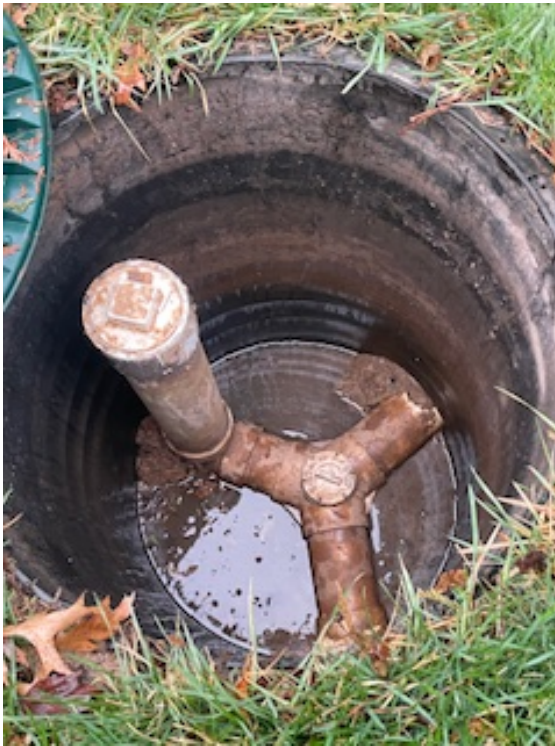
Bull run valve should be replaced with 4" ball valves
