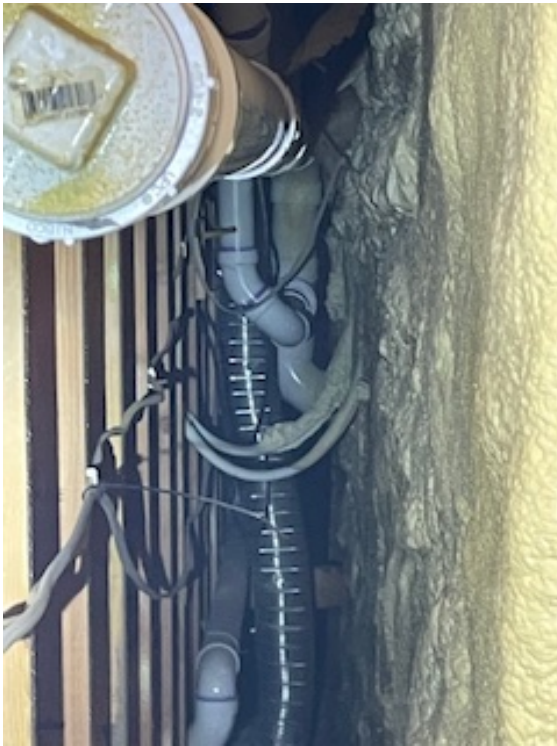
Main sewer line out basement wall
