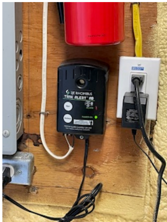
Holding tank alarm control panel
