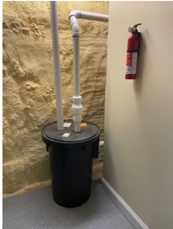
Washer pump station
