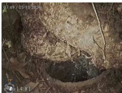
Showing drywell 3 observation port obstructed by the tree
