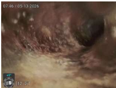
Inside cast iron sewer line from the tank towards the house, bend in line
