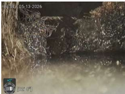
Line entering the distribution box. Root intrusion observed
