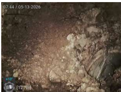
Inside the corroded and broken distribution box. When locating the distribution box probe went easily through the dbox
