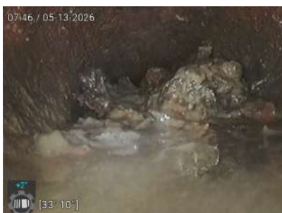
Inside cast iron sewer line from the tank towards the house. Solids buildup in sewer line
